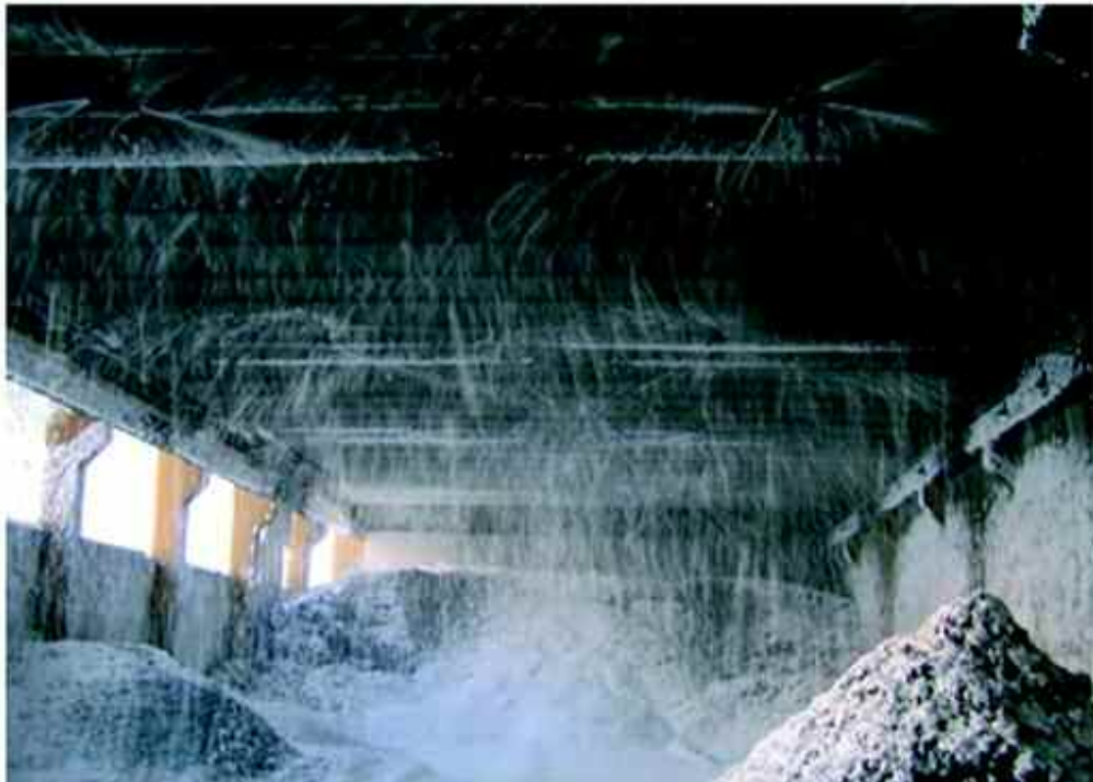
ONE SEVEN Extinction system for automatic fire fighting in a storage hall for recycling products
