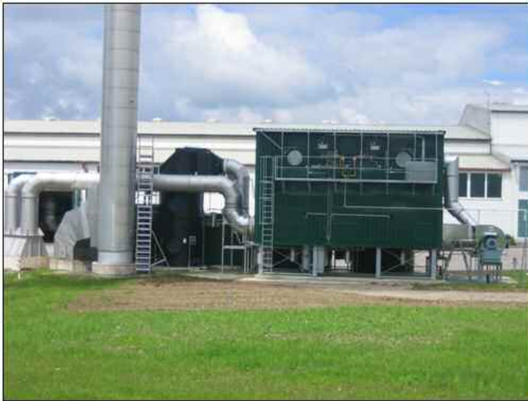
Figure 1: RTO plant with scrubber
