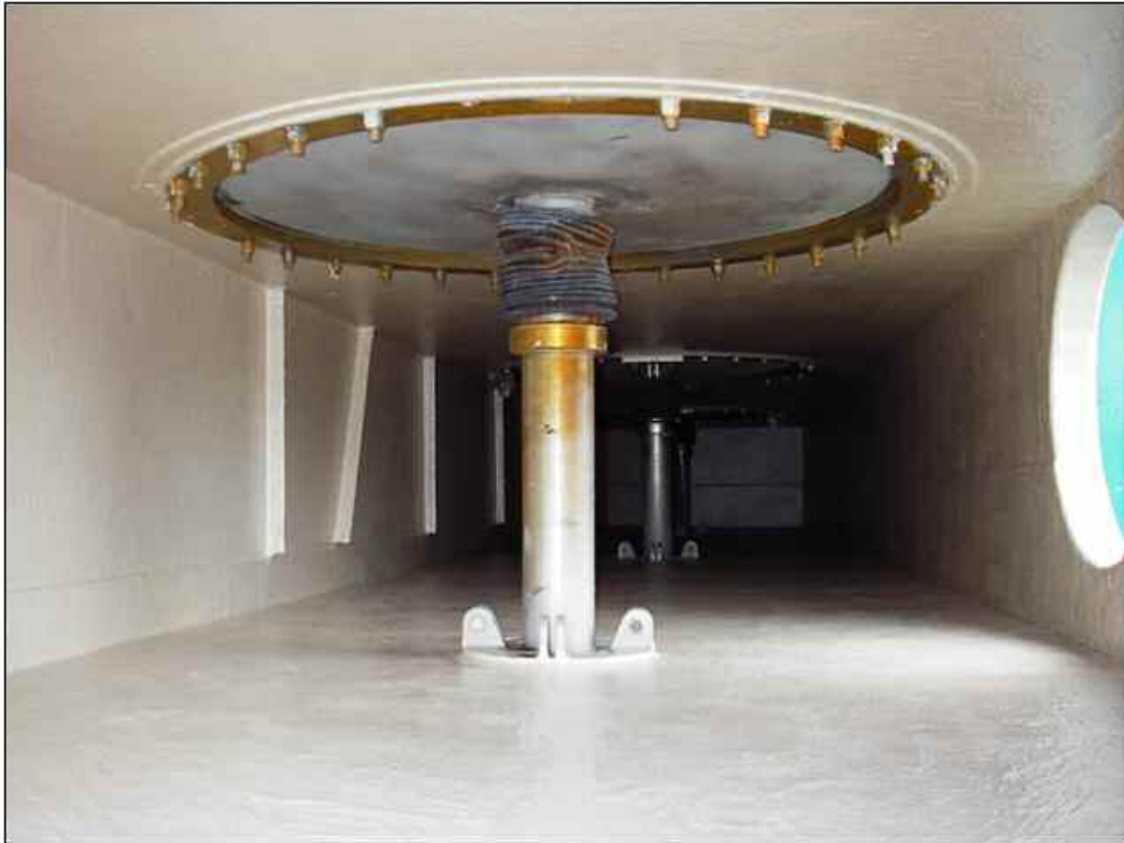
Figure 5: Re-engineered dirty gas canal
