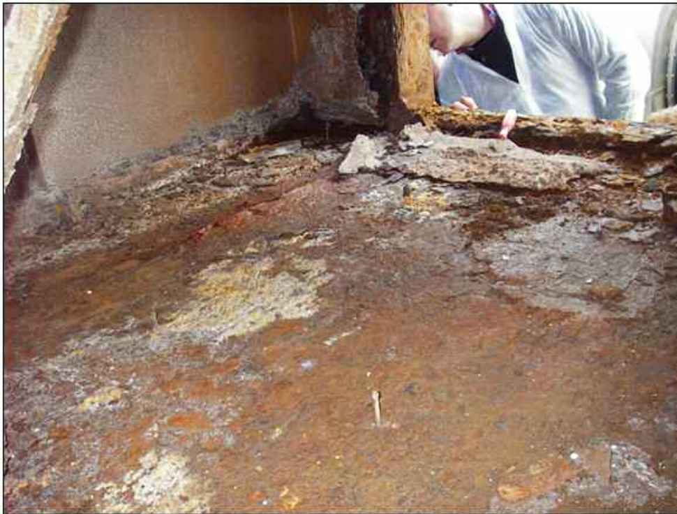
Figure 4: Corrosion in the dirty gas canal
